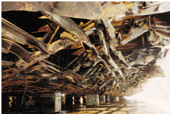
Fig. 12: Extensive tearing of the bottom plate of a single hull tanker under grounding action.
